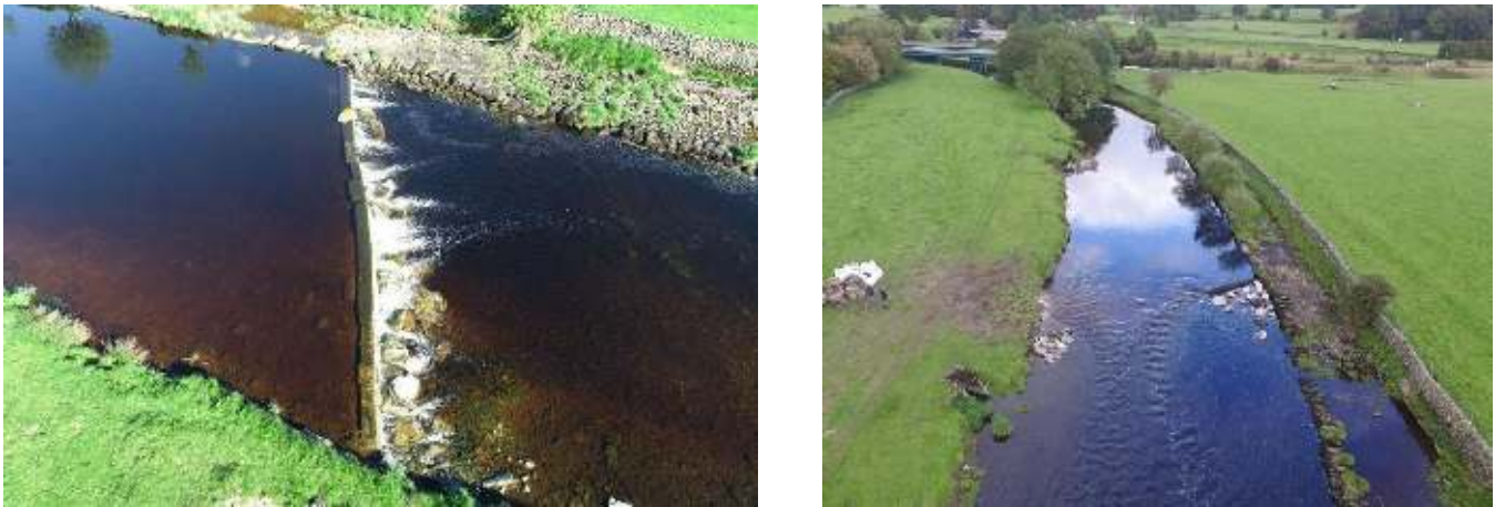
Figure 4.0.3. Partial weir removal on the River Ribble adjacent to Settle sewage works
