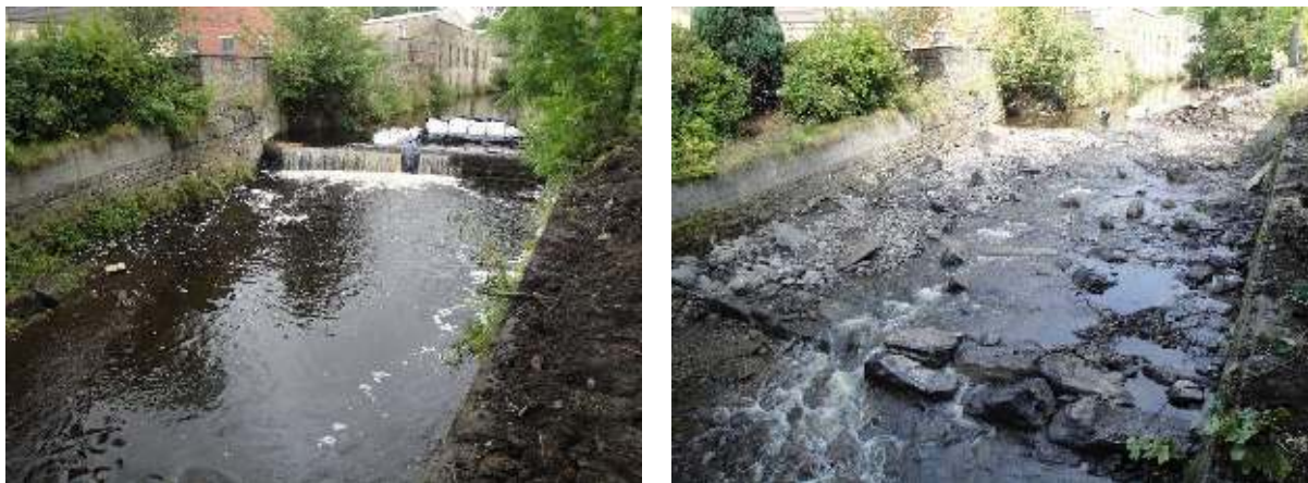
Figure 12 Before (left) and after (right) photos of a fish passage solution on one of the weirs along Colne Water. One of five easements adult salmon would have had to ascended to spawn.
