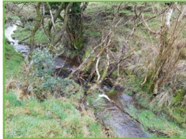
Images left: Leaky dams were constructed from stakes and locally sourced branches
