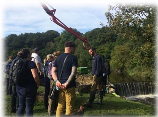
Project Manager Adam Walmsley talking participants through the construction of Dunkenhalgh fish pass on the Hyndburn Brook walk
